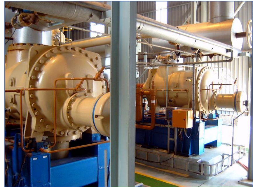
Howden WRV 322 Ammonia Compressors
