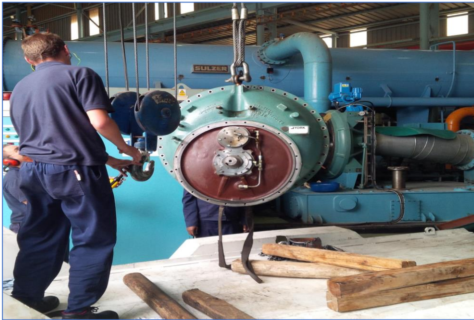
Sulzer Plant with York YK J4 Compressors
