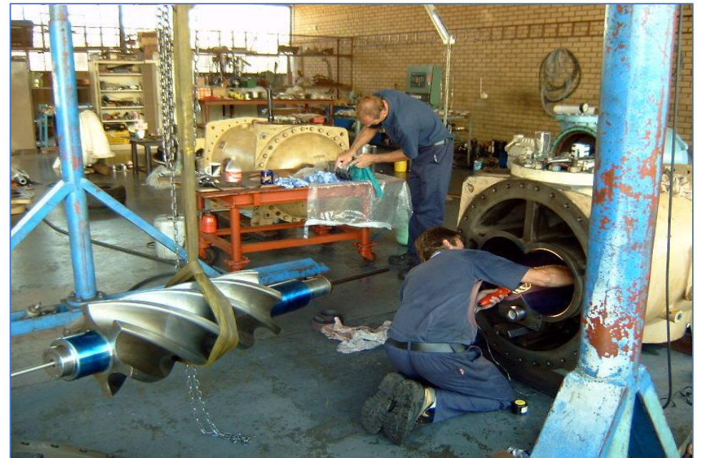
Howden Ammonia Compressor
