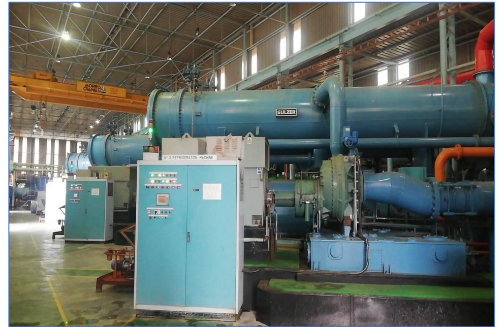
5 X Sulzer Plant with York Yk J 4 Compressors
