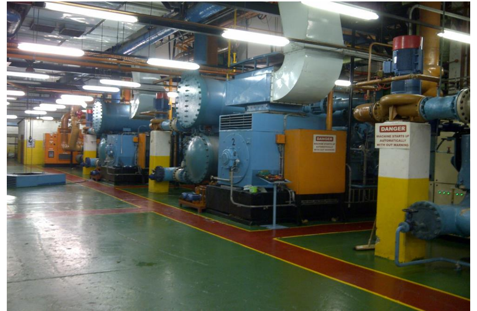
York Multi stage 238 Compressor Chillers
